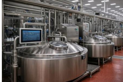
Dairy & Beverage Production Line
